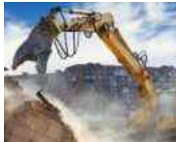
Dust from demolition sites
